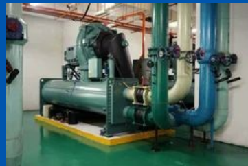
Water Chiller Plant
